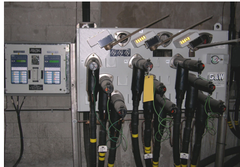
Vault switch with SEL controls.
