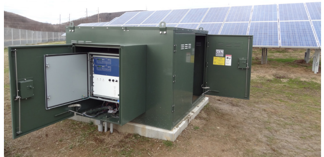
Padmount switch with SEL controls.
