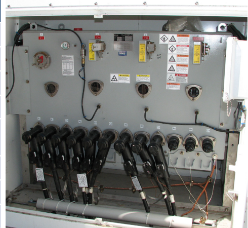
Front access PNI with load break rotary operator and interrupter single operating handle.
